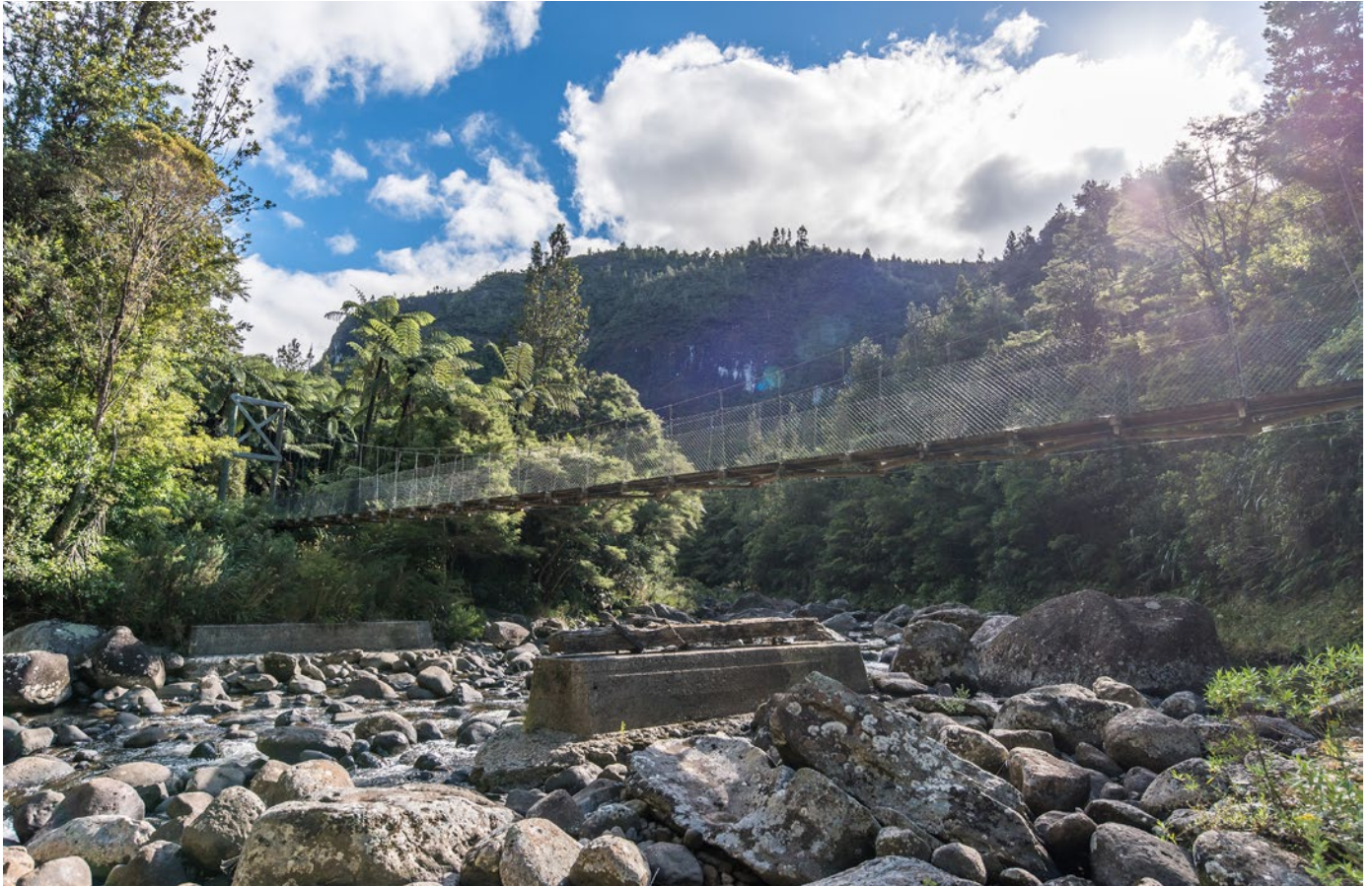
Figure 3.11: The ‘impassable’ crossing point. The concrete foundations are all that remain of the old tramway bridge. (Source: author.)
