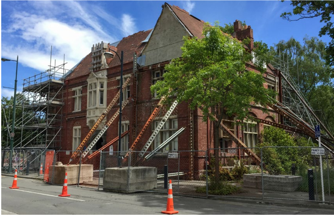
Figure 4.4: Our City O-Tautahi, an important heritage-listed building in the city centre damaged by the earthquakes. Heavily braced with scaffolding, it awaits extensive repair. (Source: Author.)
